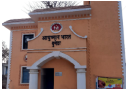
Renovating the Health and Wellness center at Dunetha, Daman for the local community.
